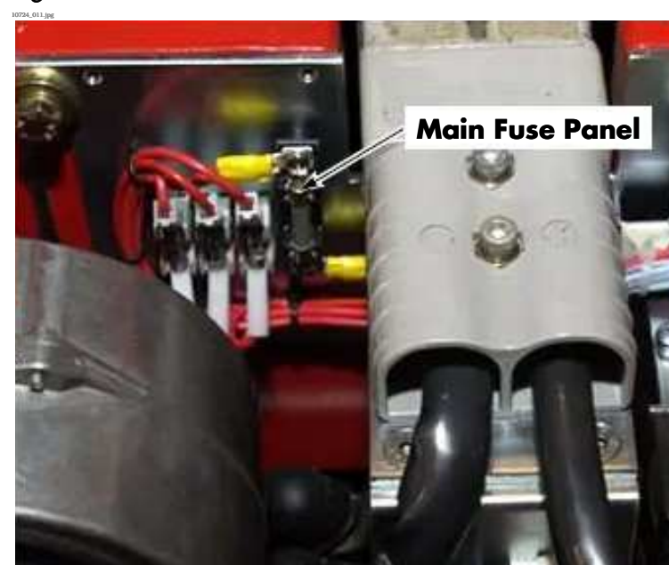
Figure 7-37. Main Fuse Panel
