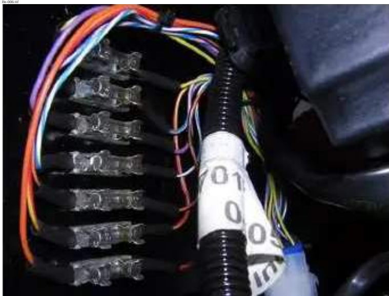
Figure 7-39. Fuse Panel Near Hydraulic Control Board
