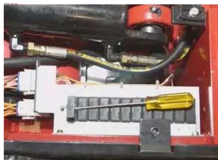
Figure 7-38. +24V Fuse Panel
