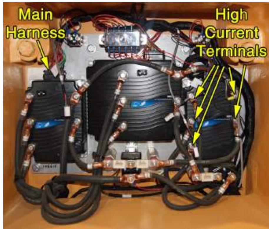
Figure 3-20: Control Panel Wiring
