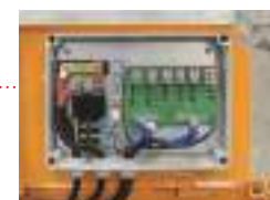
▶ Electric Control System
