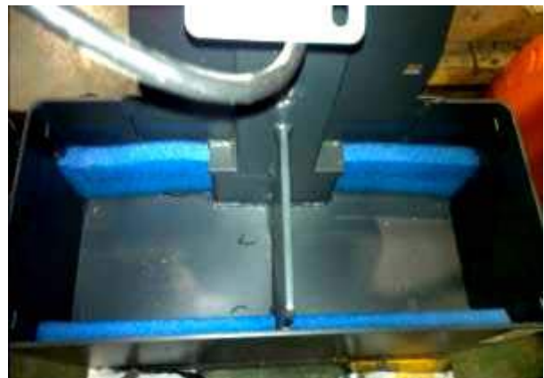
After dismantle the battery
