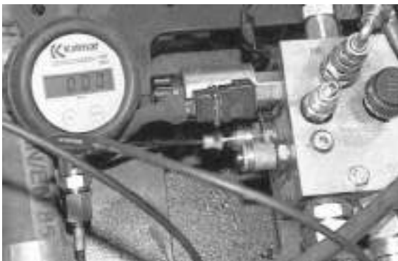
Measuring outlet, accumulator pressure
