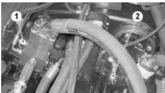
Measuring outlet, hydraulic oil pumps
