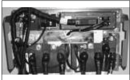
Main Fuse – 700 amps
