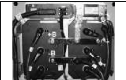
Main Fuse - 800 amps
